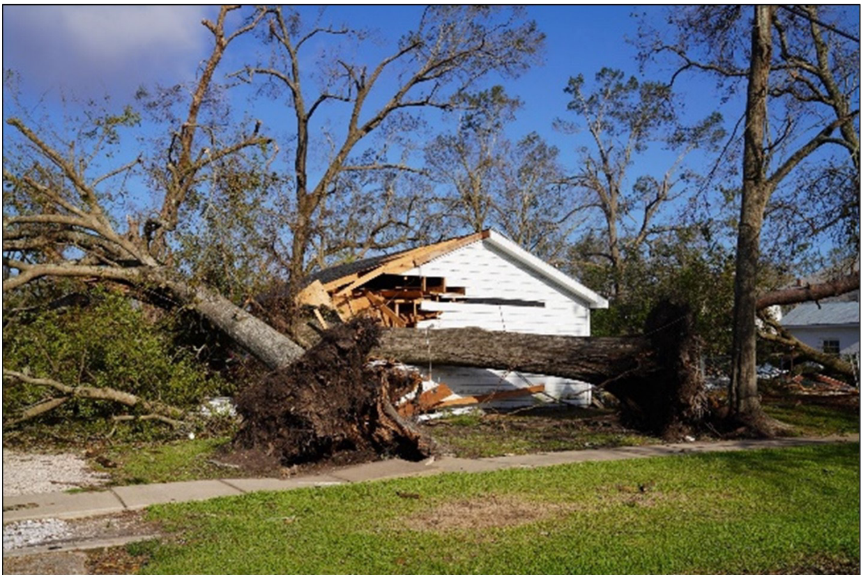
Figure 1. Severe Damage to a Home in Lake Charles, LA, Caused by a Fallen Tree During Hurricane Laura, Observed on August 29, 2020
